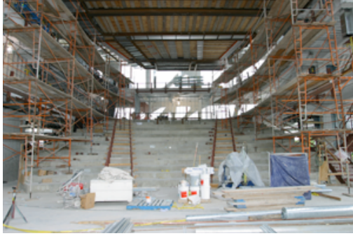
Construction of the McGuire Theater, June 2004 Photo: Cameron Wittig for Walker Art Center
